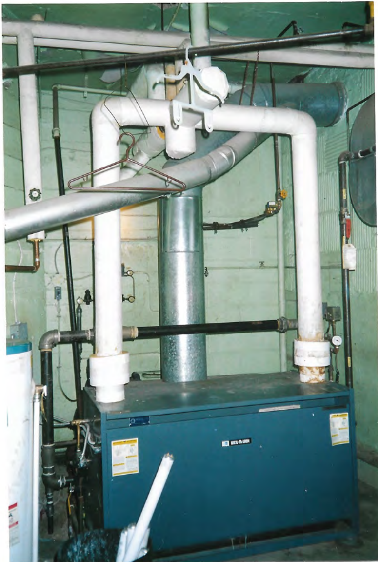
Figure 42 Welland Public Library, original library Lower level, furnace room
