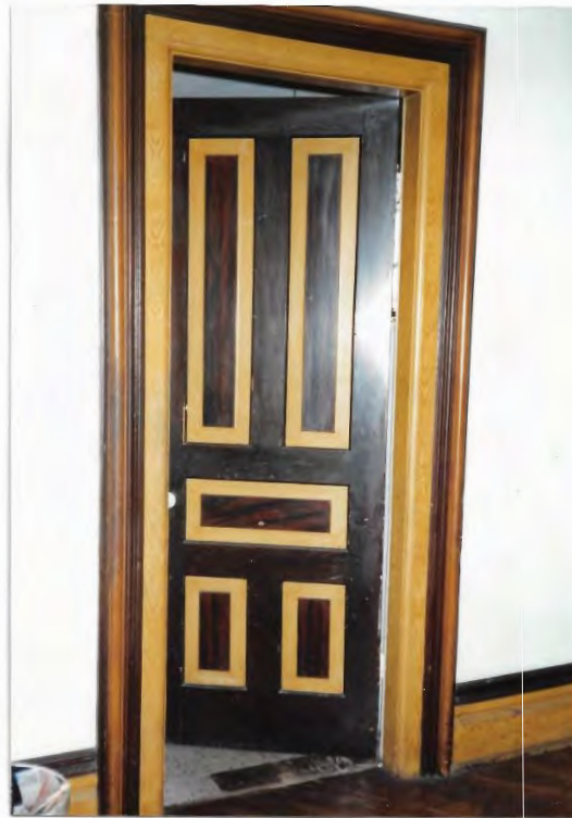
FIGURE 66 DOOR BETWEEN DINING ROOM + KITCHEN (FROM DINING ROOM) (PAINT GRAINED) WEST WING
