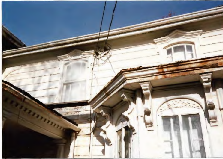
FIGURE 10 EAST WING - DETAIL OF EAVES, UPPER WINDOWS AND LOWER BAY, FRONT (SOUTH) FACADE
