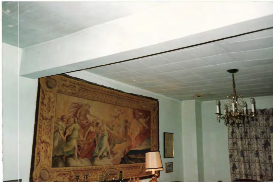
FIGURE 18 EAST WING - DINING ROOM CEILING SHOWING LARGE CENTRAL BEAM BETWEEN LIVING AND DINING ROOMS
