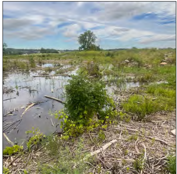
Image 40: Exposed disturbed soils and grading.
