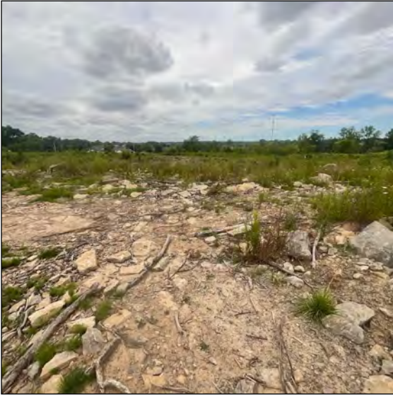
Image 41: Exposed disturbed soils and grading.
