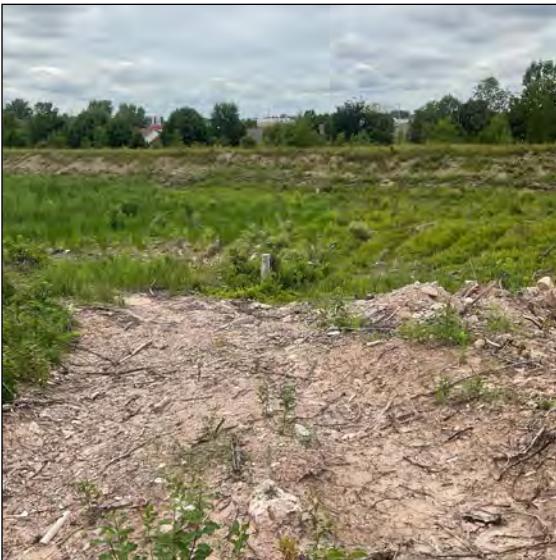
Image 31: Exposed disturbed soils and grading.
