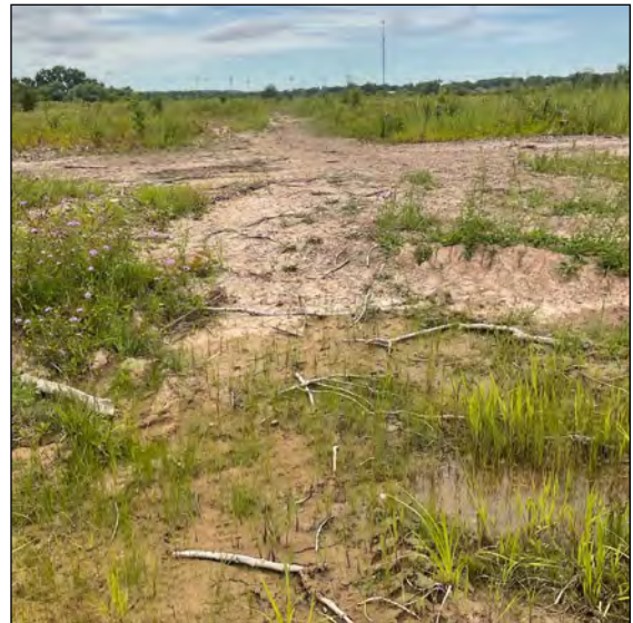
Image 36: Exposed disturbed soils and grading.
