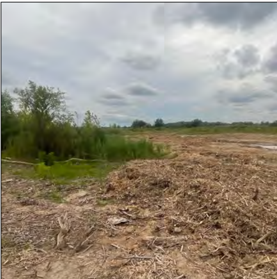
Image 43: Exposed disturbed soils and grading.
